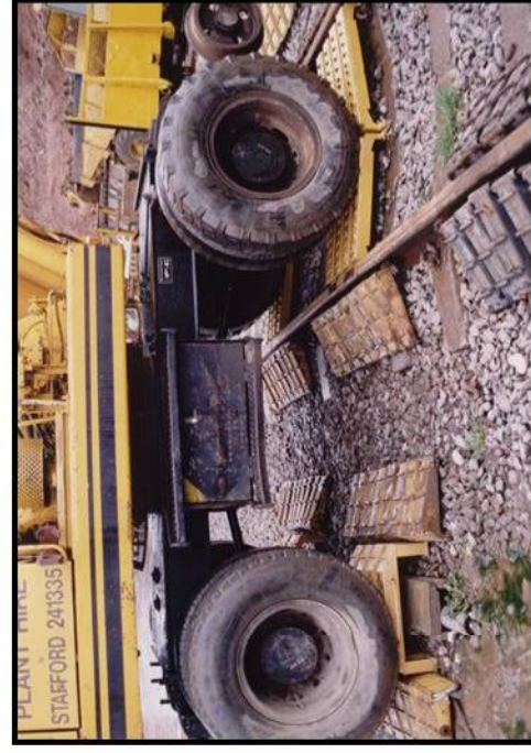
This photo shows an O&K road rail excavator safely crossing the rail and adjacent troughing.
